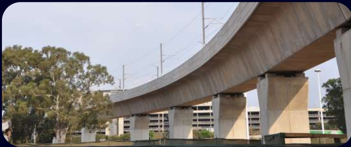
Bombardier - GAUTRAIN - Design of Gautrain bridge substructures along the southern line (Johannesburg International Airport to Midrand)
