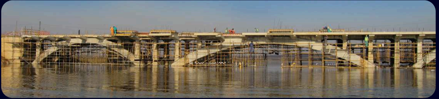
Mpumalanga Provincial Government - Department of Roads & Transport: Structural Repair of Bridge BN998 on Road P120/1 (Fulton's Commendation Award) part of the GFIP projects
